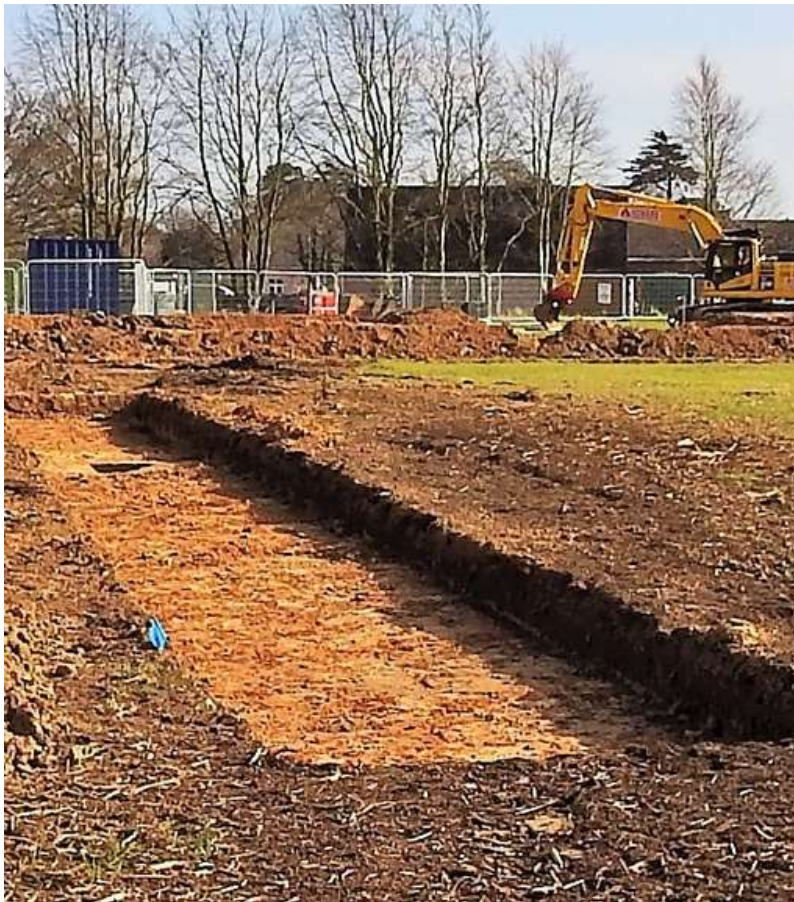
Another trench ( The light 'sandy' section, is probably a 'modern' pipe trench ?)
